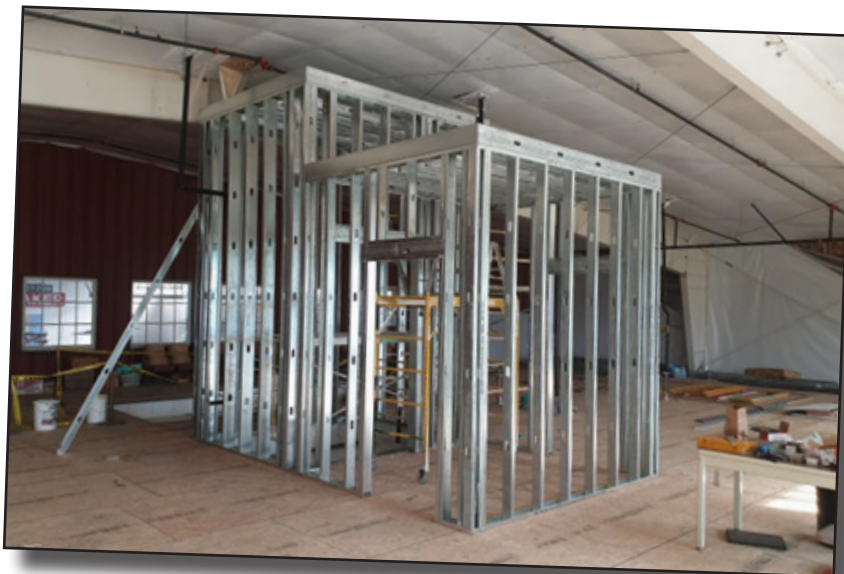
The framing for the elevator is in on the 2nd floor, and ready for the next step toward not needing steps!
